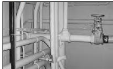
Piping and plumbing systems
